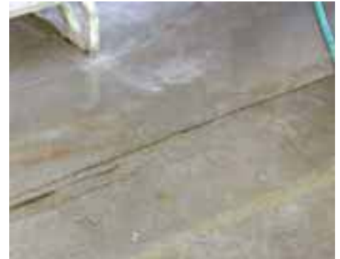
After 60 days of treatment, the area floors were clean and slight remaining scale was soft and powdery.
